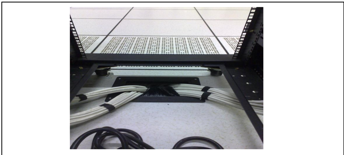
Rajah 7.4 : Cable Opening
